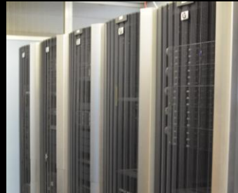
High Level Controls (HLC)
